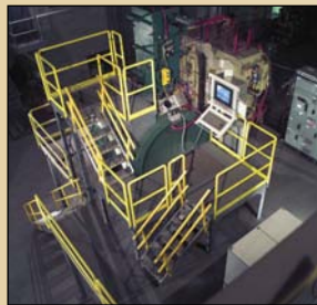
Precision casting furnace typical for SX/DX or Equiax systems
