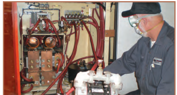
Using Magne-Clean and specialized recirculating equipment, our technician flushes deposits from the I.D. of each power supply cooling path one at a time.
