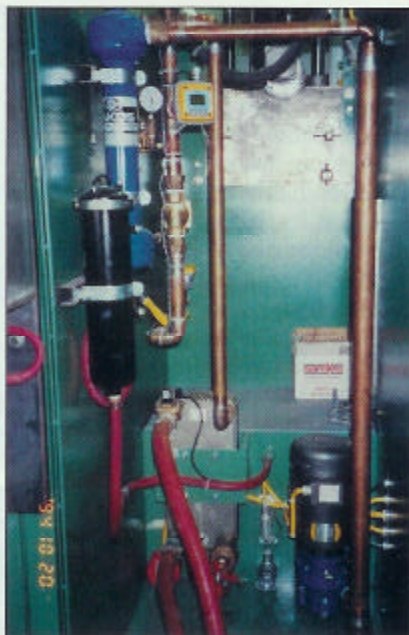
Fig. 4 — Quenchant filtration with separator and by-pass bag filter to remove scale from quench systems.
